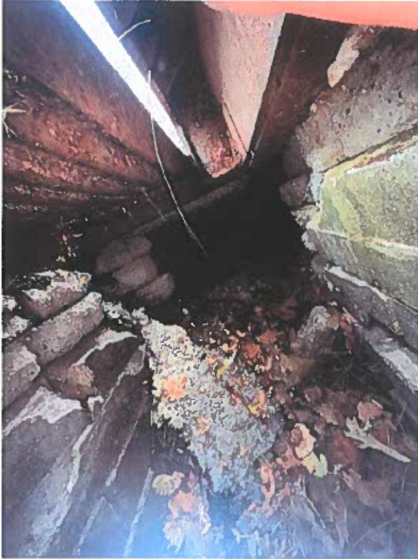
East Intake North wall blown out. – Notice void under the pavement
