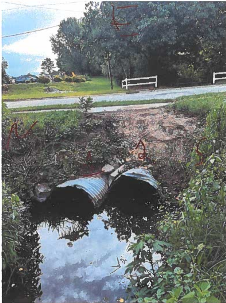
West Inlet side- Notice erosion from the sidewalk to the culverts has been filled recently.
