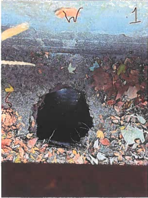
West Intake Drains Directly into Culvert Top
