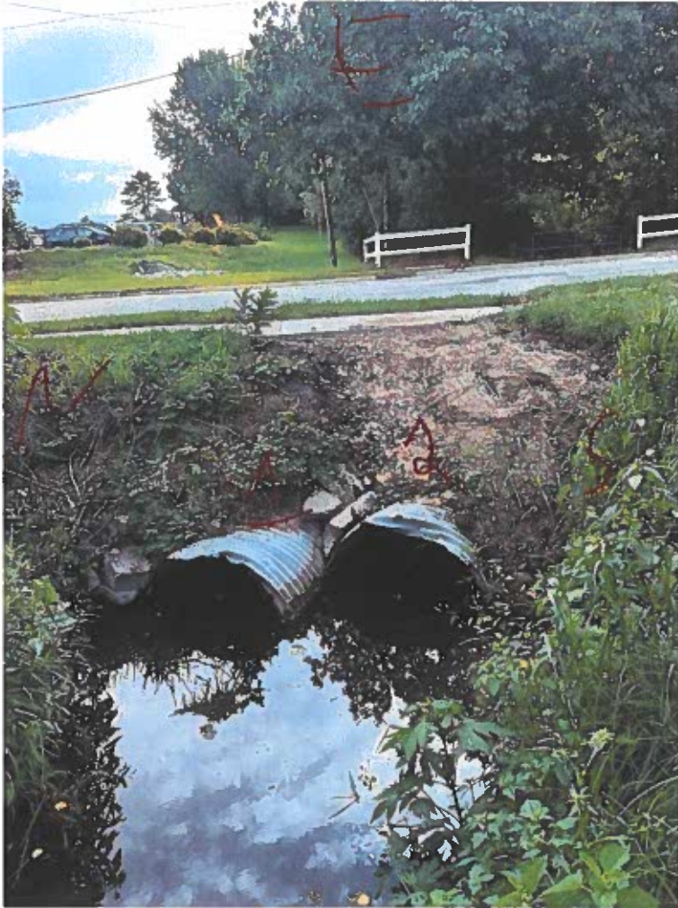
West Inlet side- Notice erosion from the sidewalk to the culverts has been filled recently.
