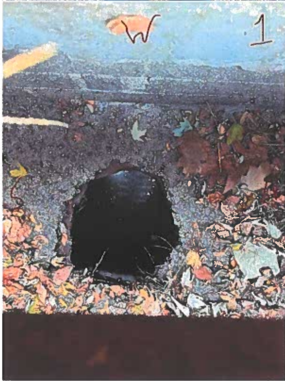
West Intake Drains Directly into Culvert Top
