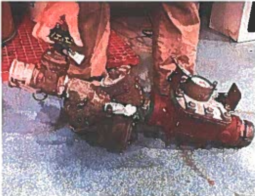
Backflow device and meter for bulk water provision at a hydrant.
