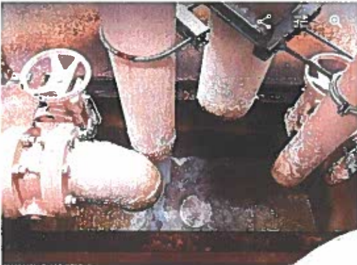
RO reject and backwash collection pit.
