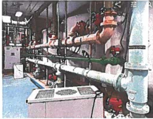
Four of the five filters & associated piping.
