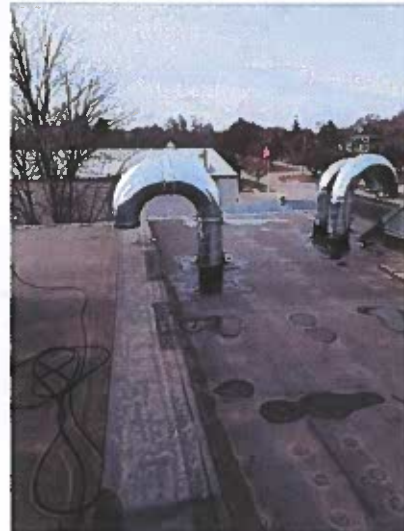
Roof – duct terminations
