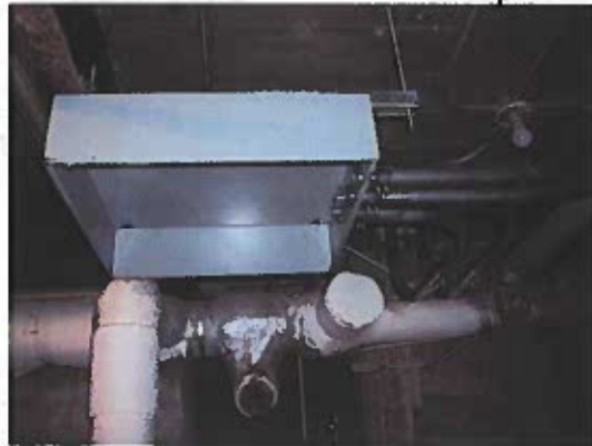
Basement – Panel D new pull box for Feeder
