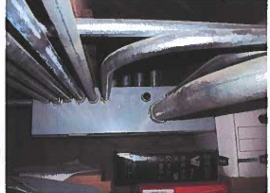
Basement – Pull Box for Panel A
