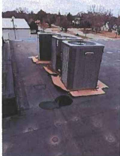
Roof – condensing units
