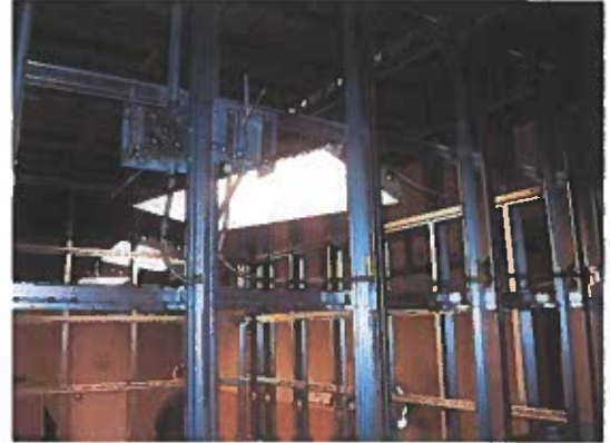
Interview 108 – MC cable to be replaced
