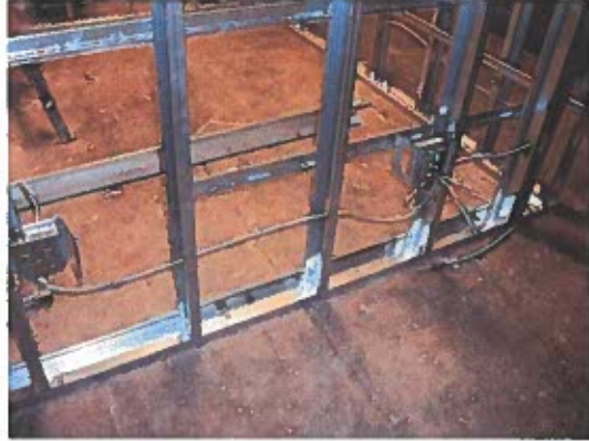
Interview 108 – MC cable to be replaced
