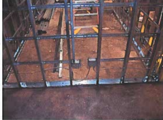
Interview 108 – MC cable to be replaced
