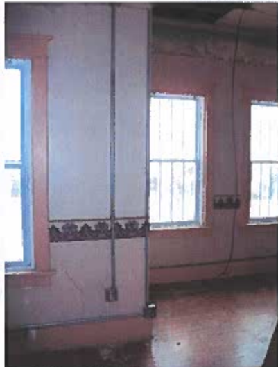
Multipurpose 201 – Conduit/box at corner to be relocated
