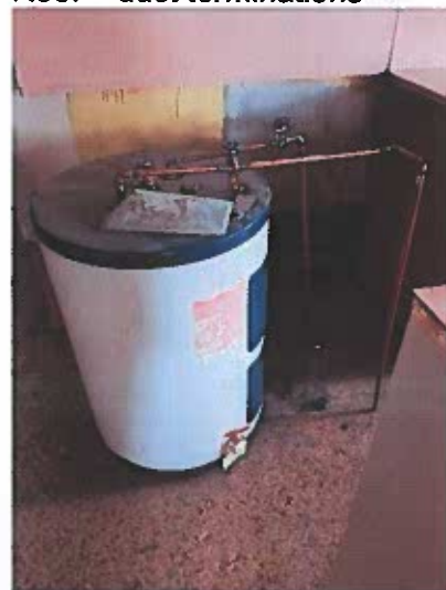
Staff Breakroom 202 – Existing water heater.
