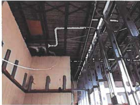
Sanitary and domestic water piping installed on first floor.
